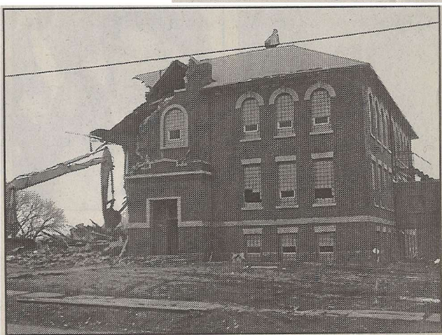
This picture taken on April 10th shows nearly one-third of the west wide of the school torn down.
