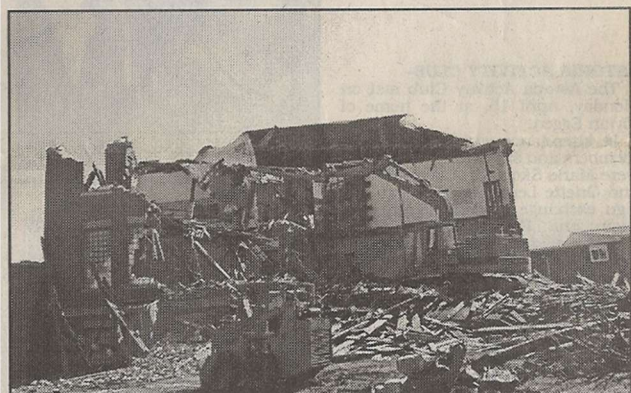
Another picture from the west side of the building with part of the northwest corner of the wall still standing.
